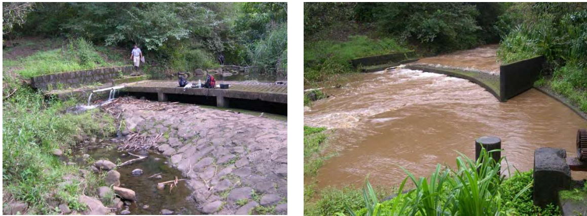
Figure 13. Two images of Honopou Stream, Maui at low (left) and high (right) flows. At low flow the barrier is a complete blockage to upstream migration and at high flow most of the water flows through the diversion structure. As postlarvae move upstream through the structure, many would be entrained in the diverted waters and removed from the stream.
